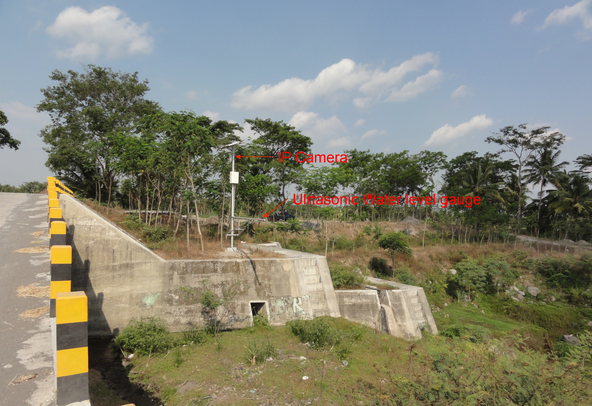
Fig.6 Water level gauge& IP Camera
